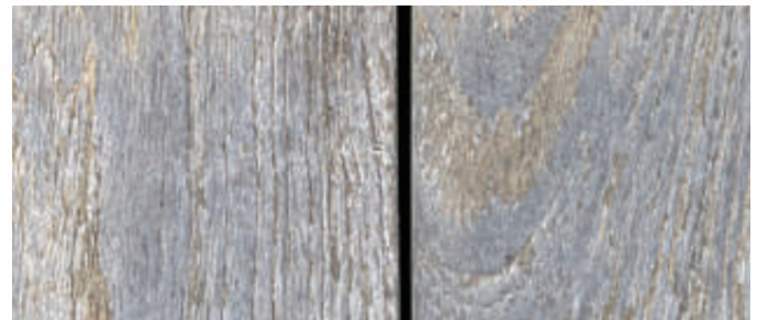
Advanced weathering (most finish worn away)
